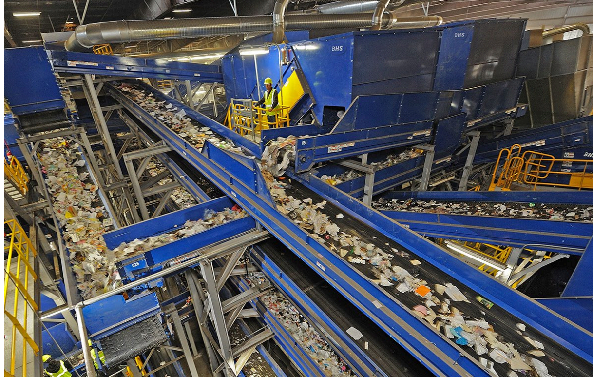
Materials Recovery Facility (MRF)
