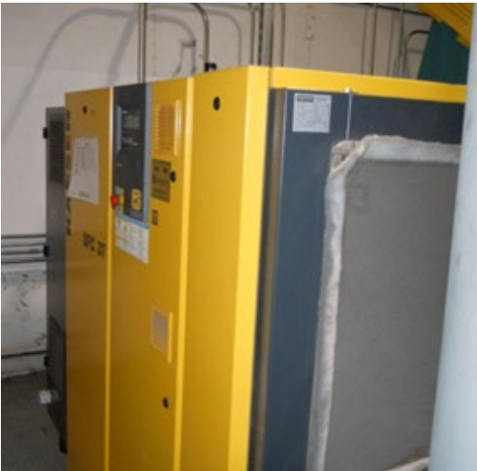
VSD air compressor
