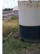
Storage tanks can leak contaminants
